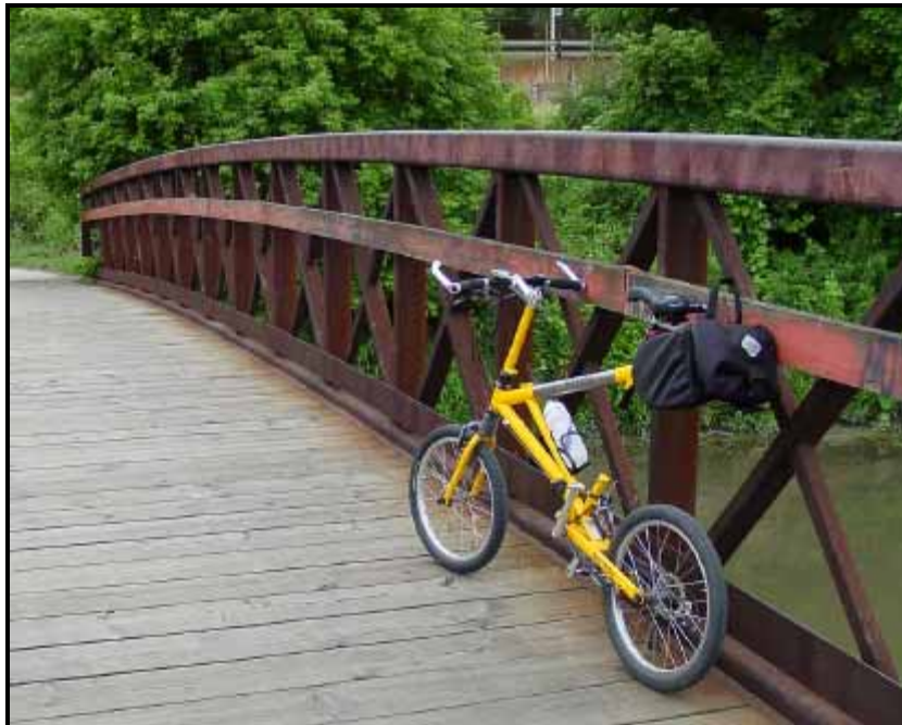
Figure 4.32 – Railing with Rub Rail (Toronto, ON)
