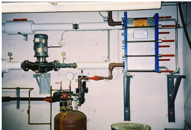
Heat exchanger transferring arena waste heat to Juan De Fuca Pool Source: Accent Refrigeration
