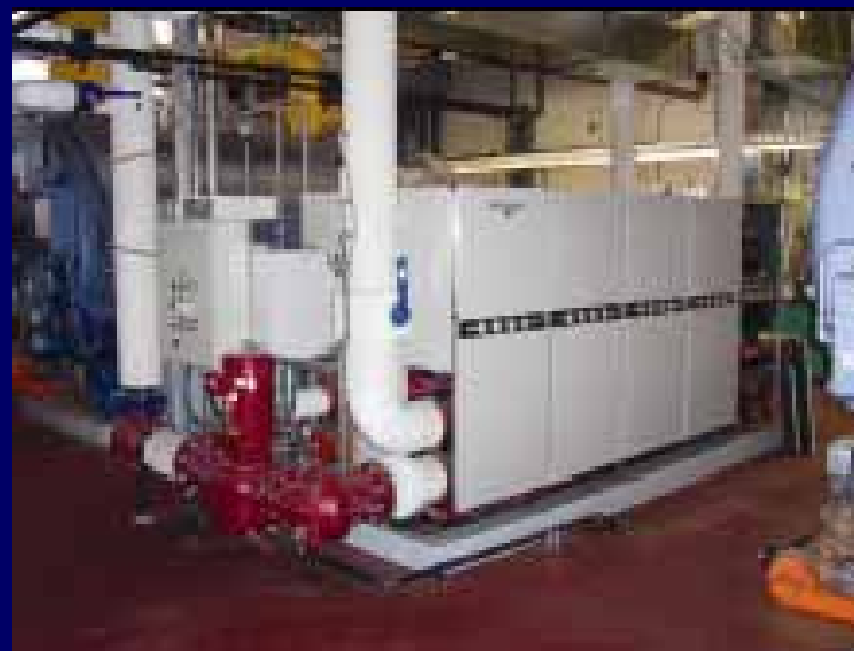
Okanagan College heat pumps
